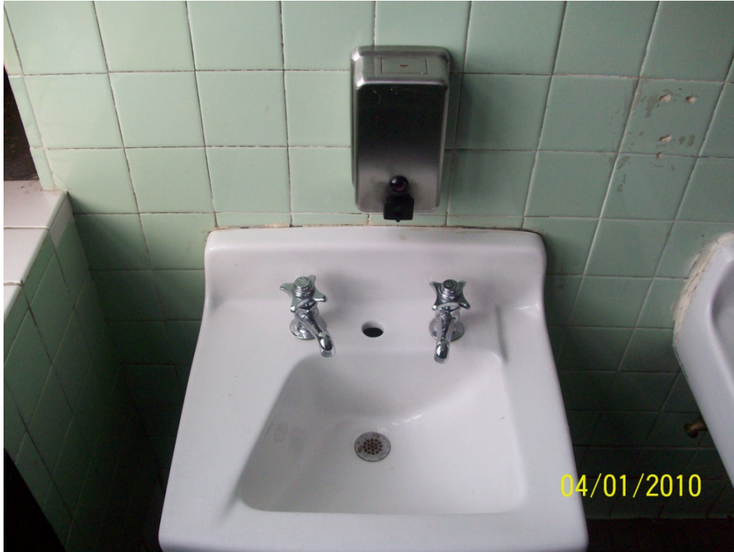
Deteriorated Sink Caulk
