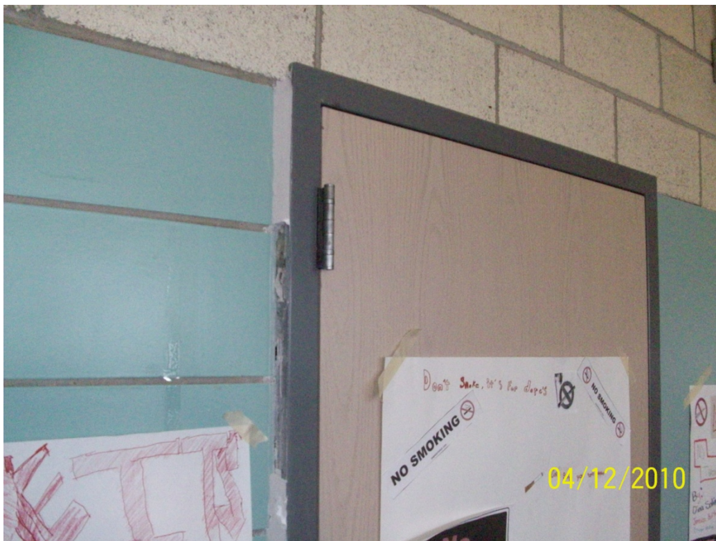
Deteriorated Door Frame Caulk
