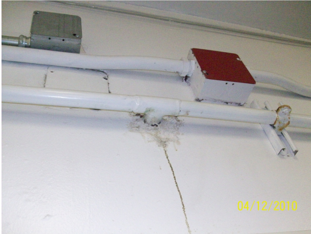
Deteriorated Fire Stop Caulk
