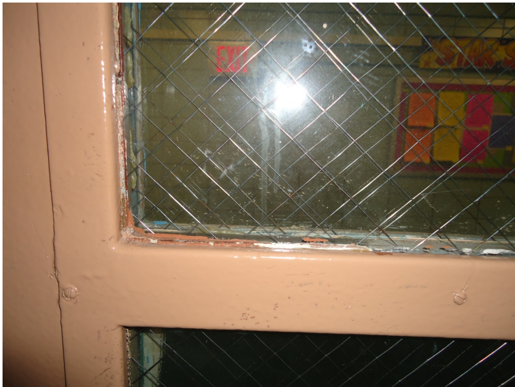
Deteriorated Door Window Glaze
