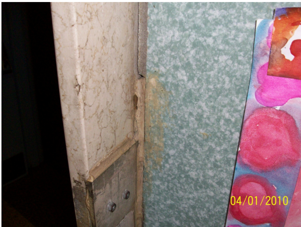
Deteriorated Marble Caulk
