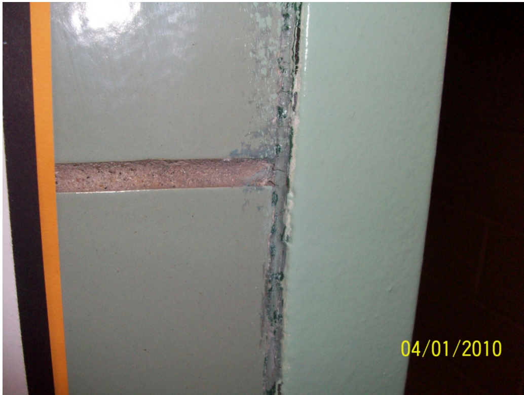
Deteriorated Door Frame Caulk
