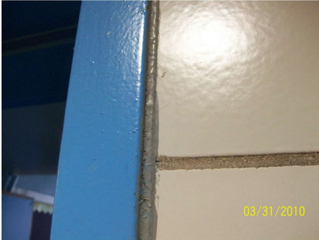
Deteriorated Door Frame Caulk
