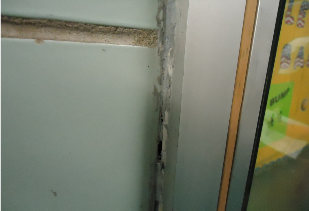
Deteriorated Display Case Caulk
