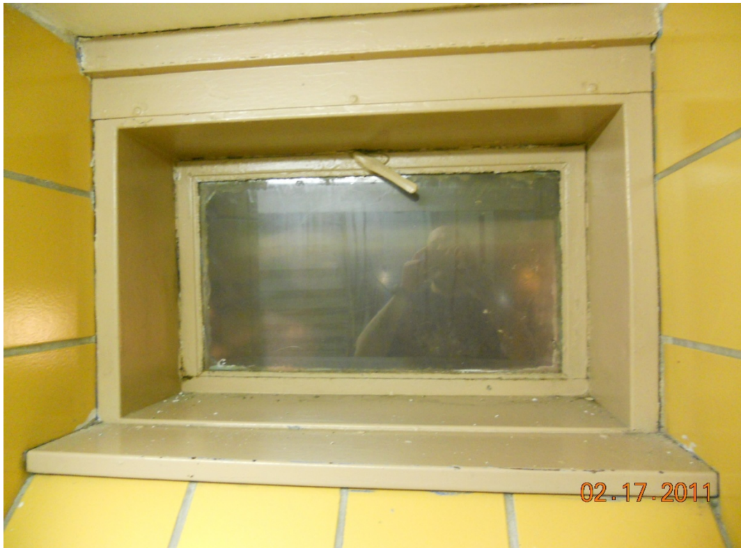
Deteriorated Window Glaze/Caulk
