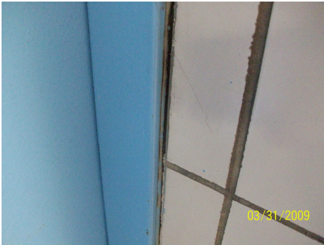
Deteriorated Door Frame Caulk
