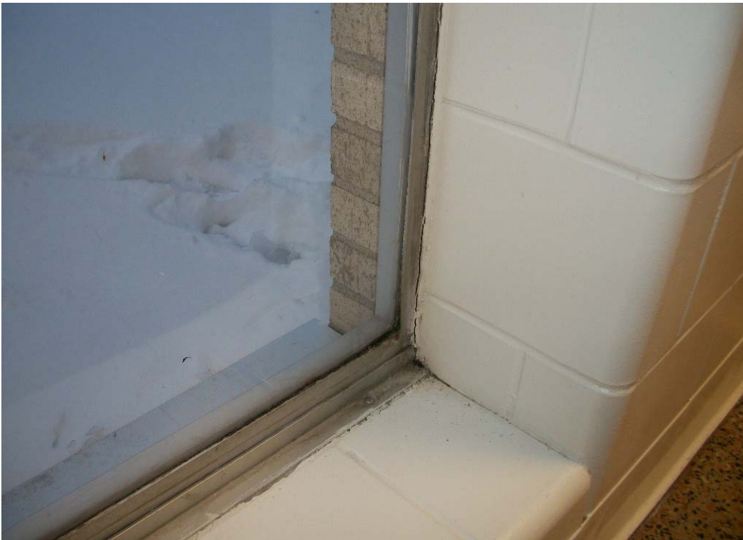
Deteriorated Window Caulk
