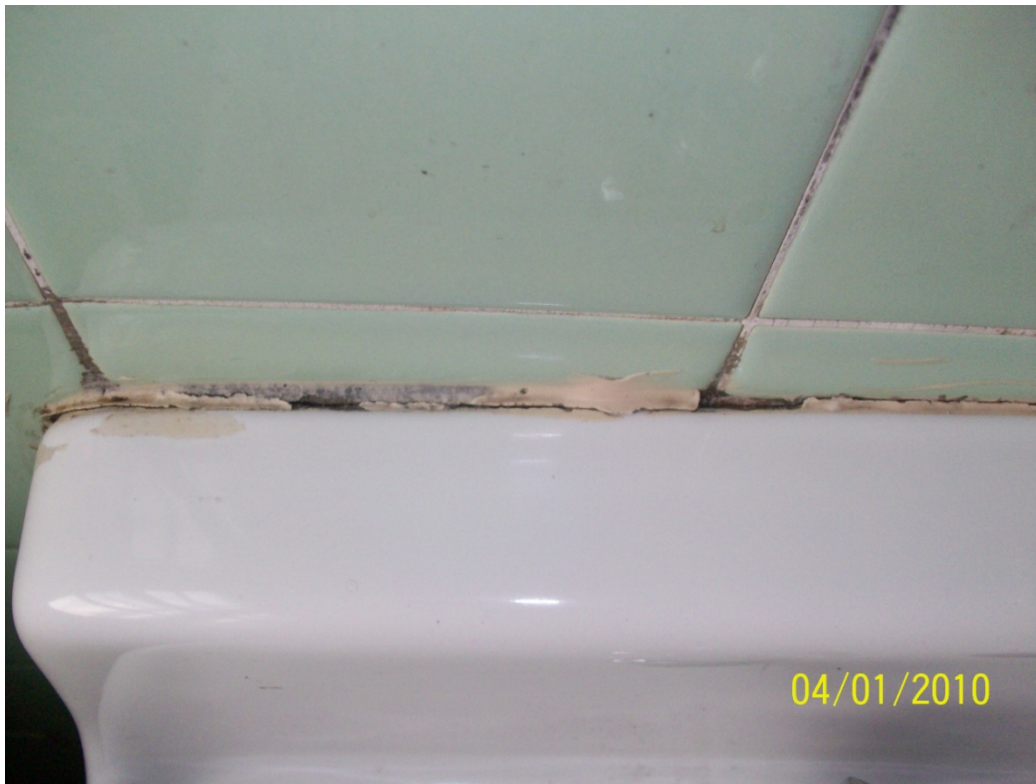
Deteriorated Caulk Close-up
