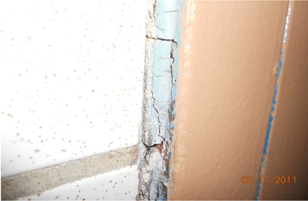
Deteriorated Caulk – Close-up
