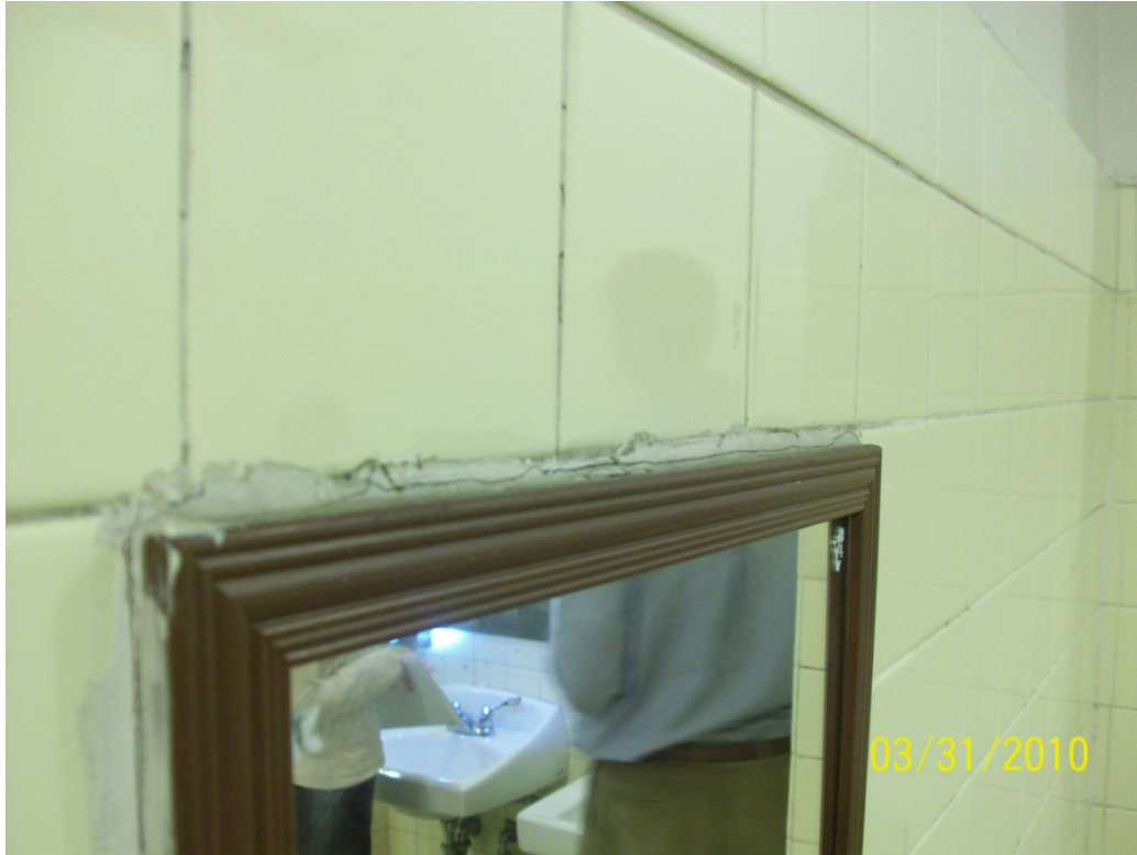
Deteriorated Mirror Caulk
